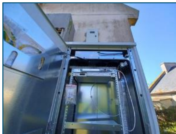
Armoire HEP installée
